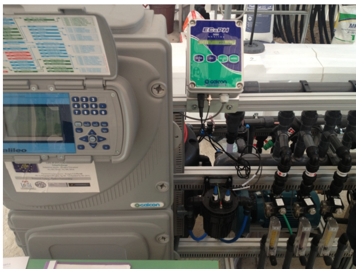
The computer of the automated hydroponic system established in Larissa
